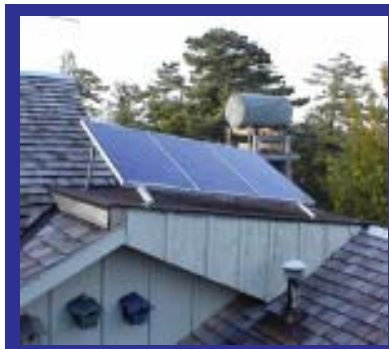
Rooftop solar can provide new energy
